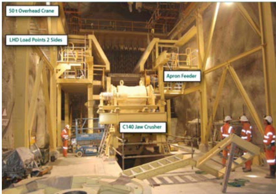
Figure 17-2: Example of a crushing station in an underground chamber
